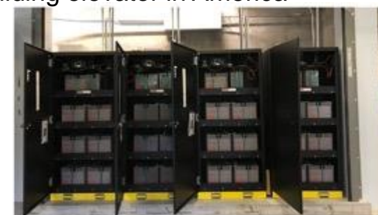
2 Hour Battery Backup
